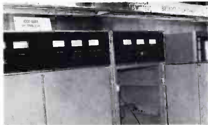
Emcee's new 1000-watt UHF translator was part of a line, from 1 watt up.
